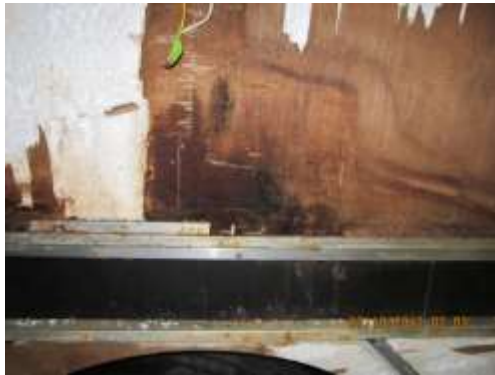
Close up of skin removal
